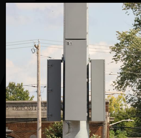
WIRE ACCESS OR POLE MOUNTED BOXES
