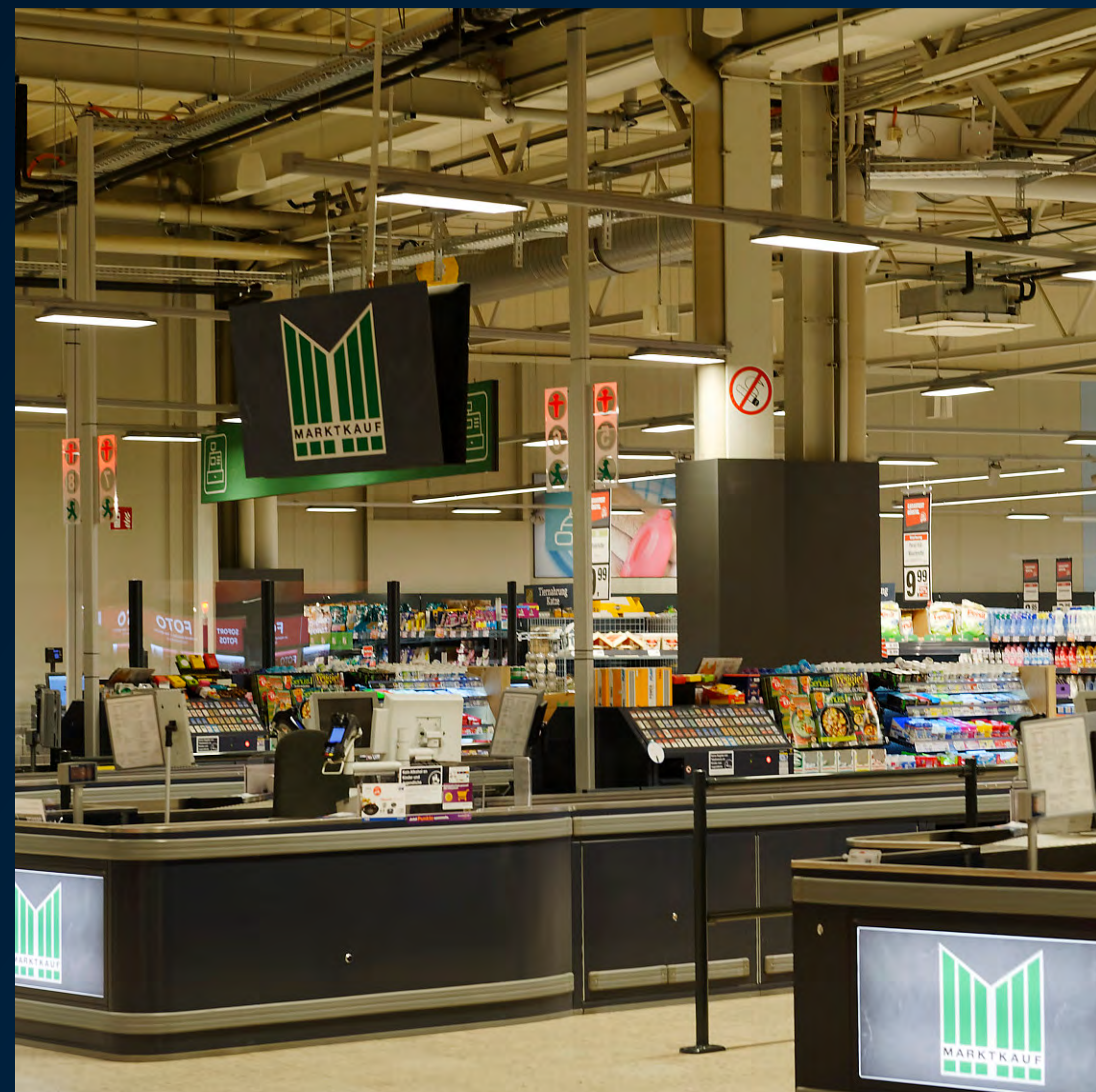
StoreSet Evo WB-OC above checkout areas reduces the risk of errors caused by distracting glare and improves comfort and productivity.
