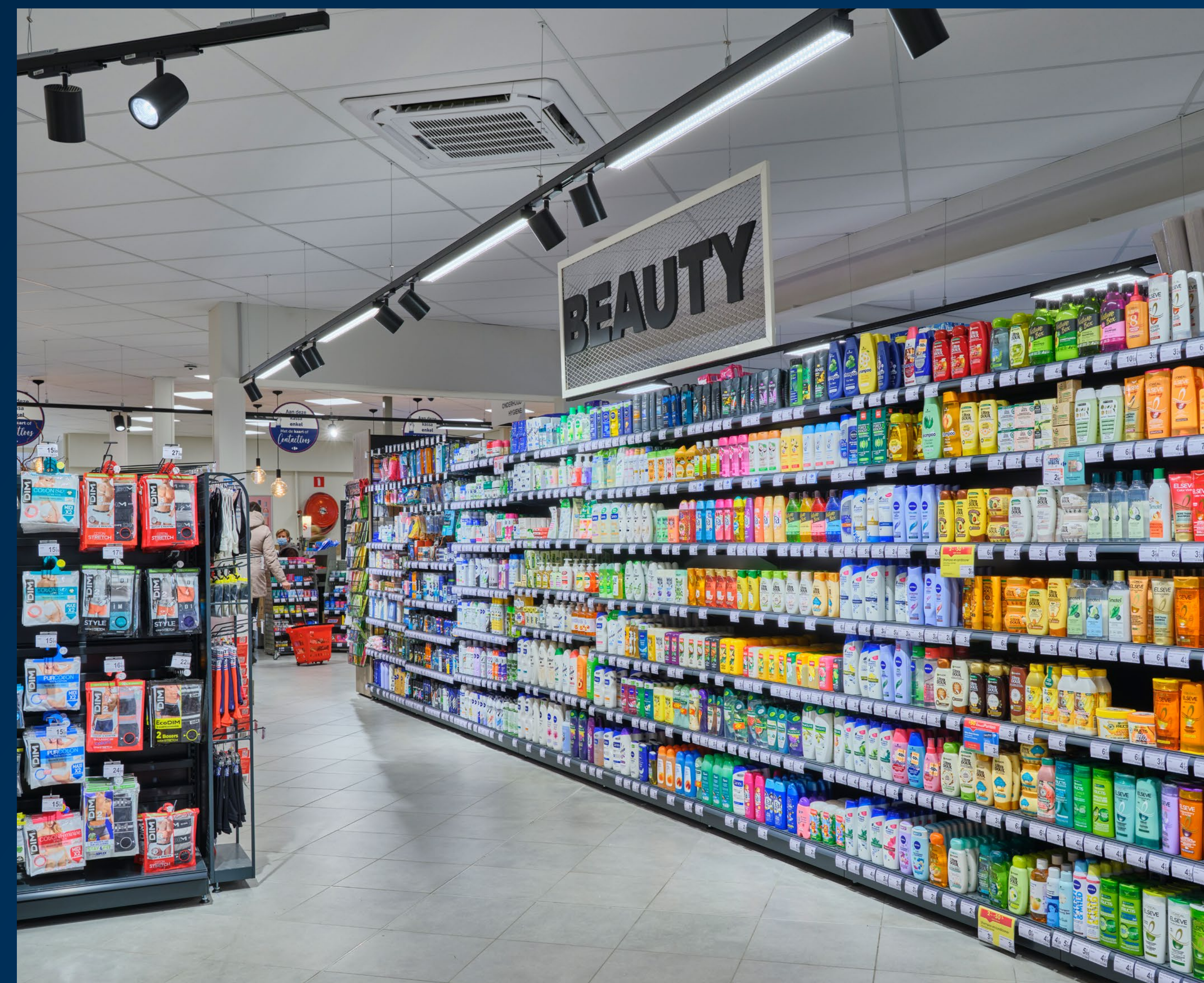
StoreSet linear combined with projectors for accent lighting, creating a lighting effect that's rich in contrast but balanced.
