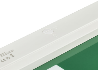
Emergency Exit Sign EM159C DET02
